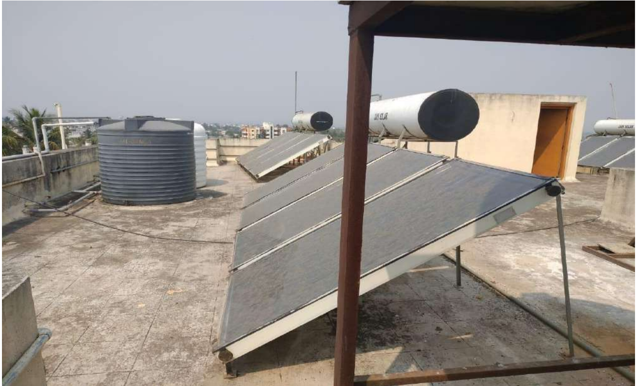
Solar Water Heater
