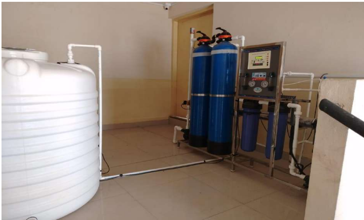
Drinking water facility (RO)
