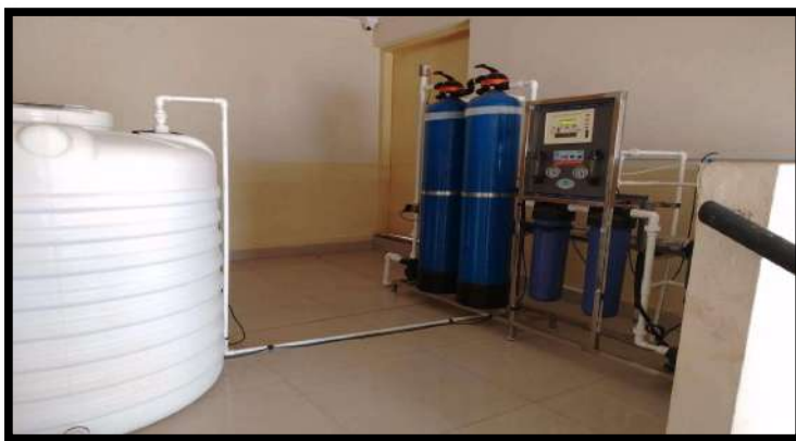
Drinking water facility (RO)
